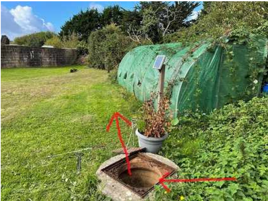
MH 5211 LOCATED IN PRIVATE GARDENS
